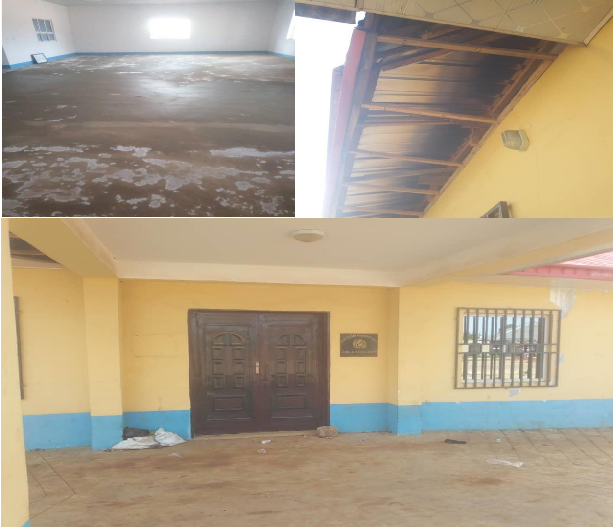
Fig. 5.2.2: Picture showing inside of the clinic room/hall with no beds or any medical equipment, water-marks on floor due to rain drops, falling ceiling boards of the Clinic; Pix below is the front of the Clinic. Source: Photo
