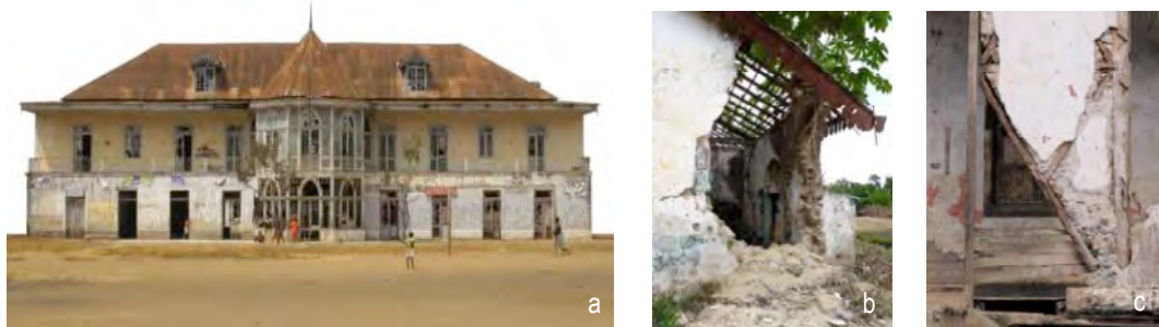
Figure 11. Example of the built heritage within the estates and their advanced state of degradation, Roça Boa Entrada, São Tomé – (a) main house, (b) warehouse, (c) technicians' house [ASF+HMS].
