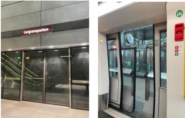
Figure 4.8 Platform Screen Doors system, Metro station in Copenhagen
