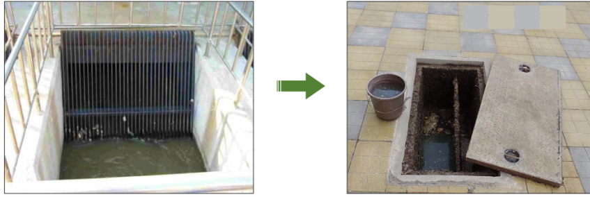
Figure 69. Chambers and oil collectorl. by: ITT Bombay.
