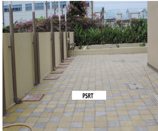
Figure 71. The surface of PSRT with access doors and odors ducts. by: ITT Bombay.
