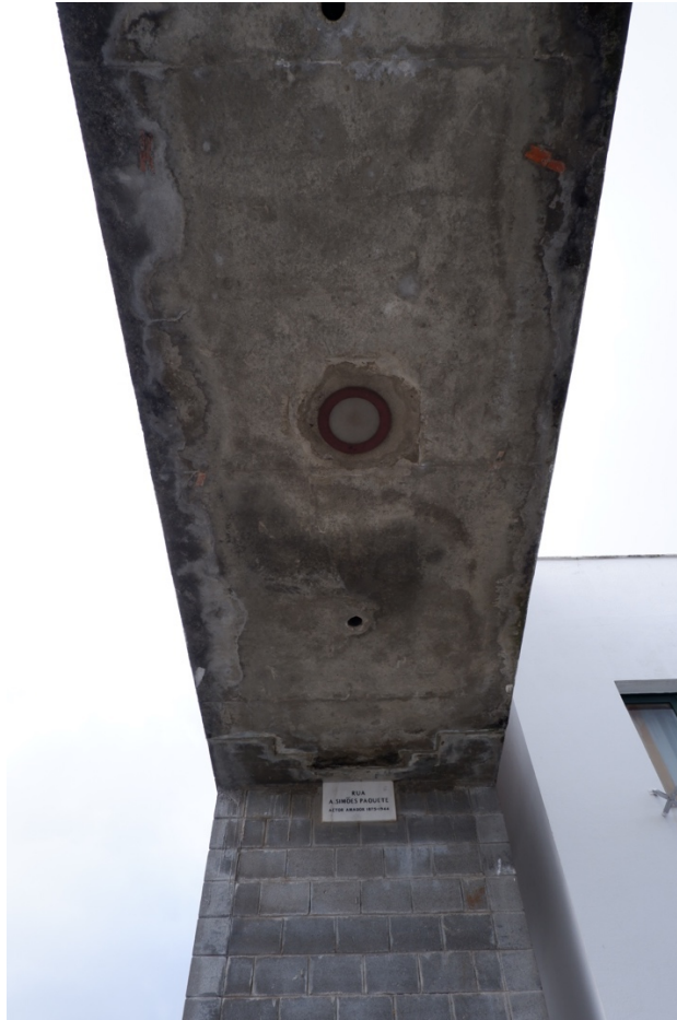
Figure 56. Water infiltration. By author.
