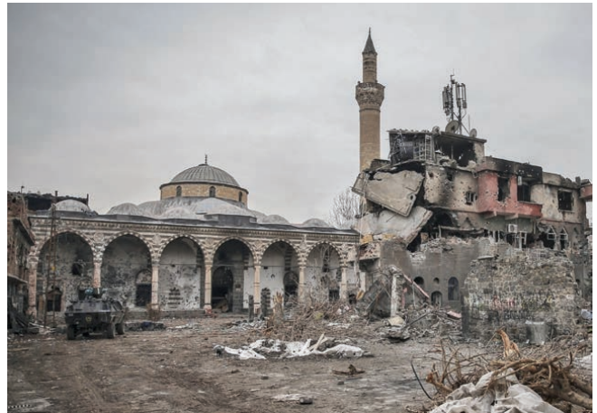
Fig. 1: The destroyed courtyard of the Kurşunlu Mosque.
