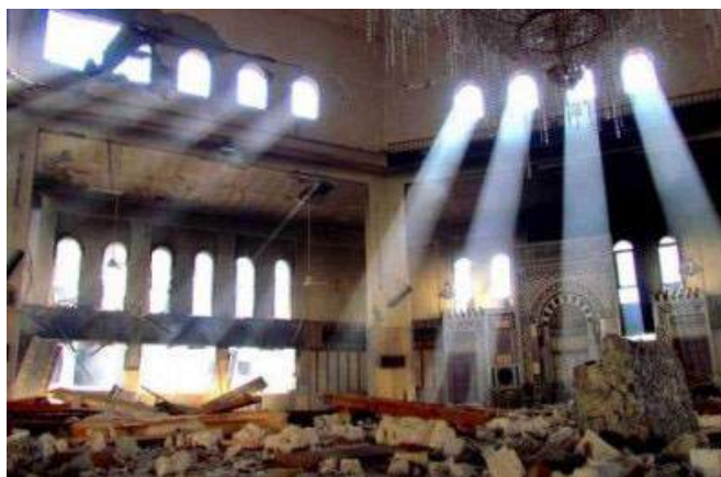
Figure 49: The destruction in the big mosque of Douma.
