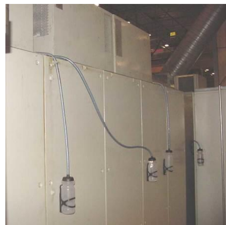
Figure 16 – Water collecting system
