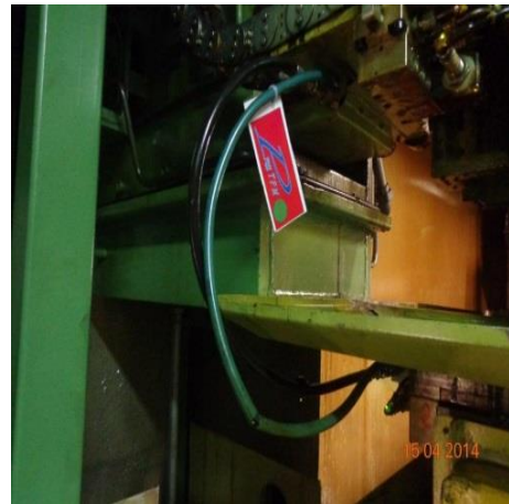
Figure 15 – Oil recycling system
