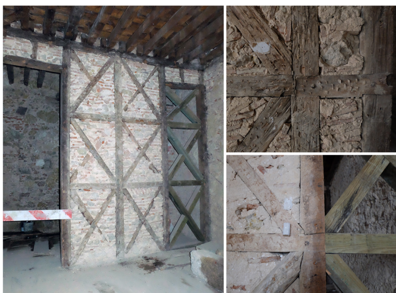
78 79 Fig. 2 – Internal view of a Pombalino building, Rua dos Fanqueiros , Lisbon (left); original 80 and replaced cross-bracing components (right)
