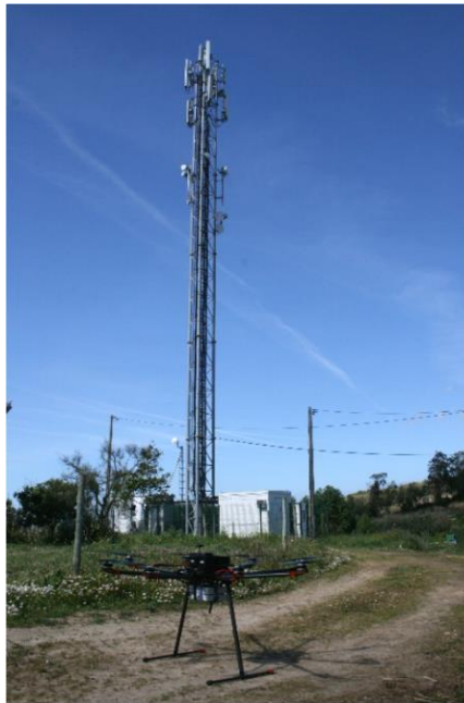
Figure 4-9. Base Station B (Vodafone)
