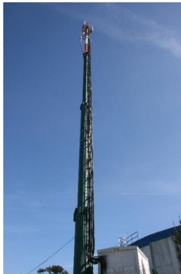
Figure 4-6. Base Station A (MEO)
