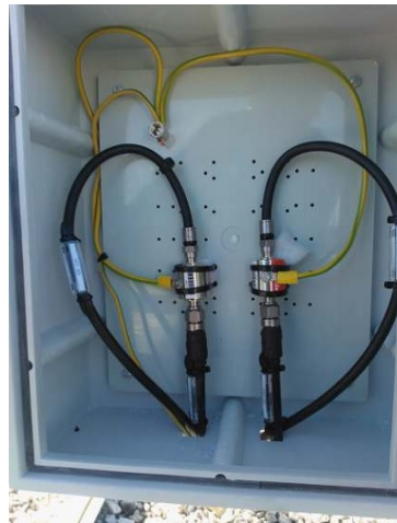
Figure 3.11: Parabolic dish lightning arrestors
