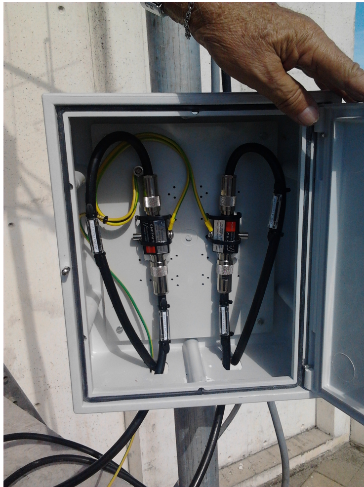
Figure 3.6: Lightning arrestors box
